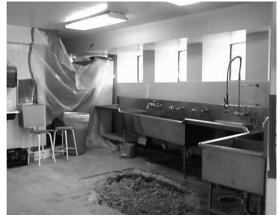
Work was recently completed on severely clogged drainpipe in the church kitchen.
